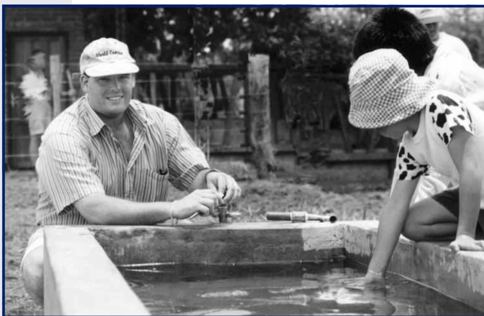
Matthew Zoller ('92), who works with World Concern on rural community development projects in Bolivia, fixes a broken water pipe on a trough for cattle. A group of local women have started a dairy, producing milk, yogurt, and butter. "Being a missionary is like being a compassionate clown," says Zoller. "We look different, talk different, have strange and funny ideas, but we long to reach the heart of the person."
